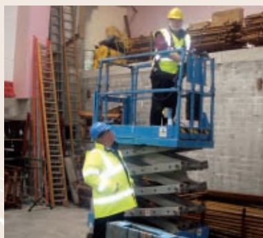
Michael O'Driscoll using the Scissor Platform under the supervision of Barry O'Donovan, HSS.
