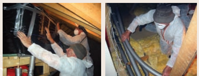
RSS Participants Con Guiney and Donie Murphy insulating pipework and a cold water tank as part of the Warmer Homes Initiative.
